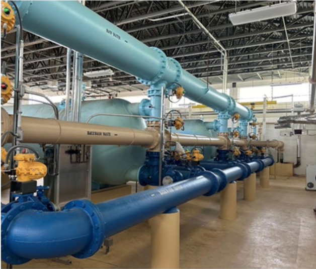
Completed in February Water Treatment Plant Valves
