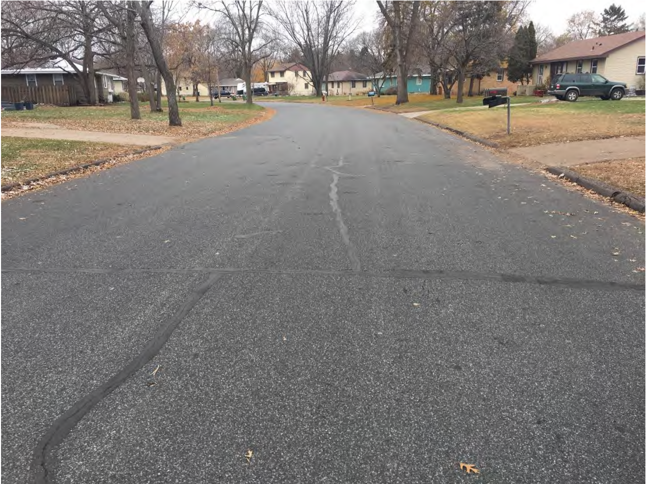
Photograph 4 – Washington Boulevard, PCI score of 70
