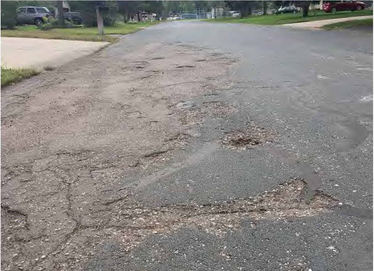
Photograph 7 – Example of Pavement Debonding with Bituminous Patching
