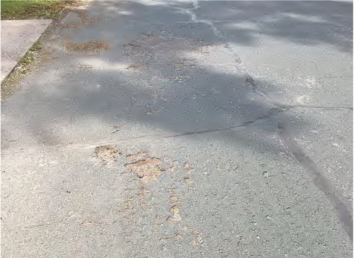
Photograph 6 – Example of Pavement Debonding
