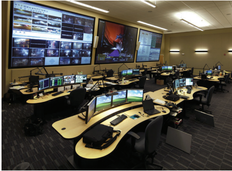
Providing situational awareness to an EOC through technology
