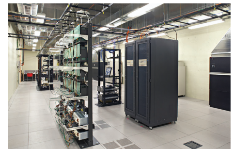
Providing hardened space for future technology flexibility and redundancy
